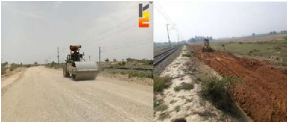
Vindhya Telelinks Limited Power Distribution Varanasi FY 2017-18
